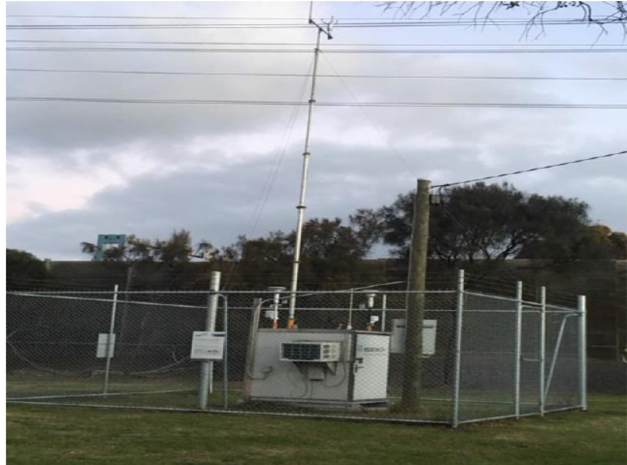
Example of air quality monitoring equipment
