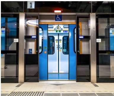
Safety first: New platform screen doors.
